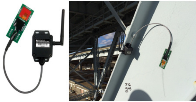
Figure 1.1. A Wireless Strain Sensor used for Real-time and Long-term Structural Health Monitoring of Bridges ( https://www.resensys.com )
