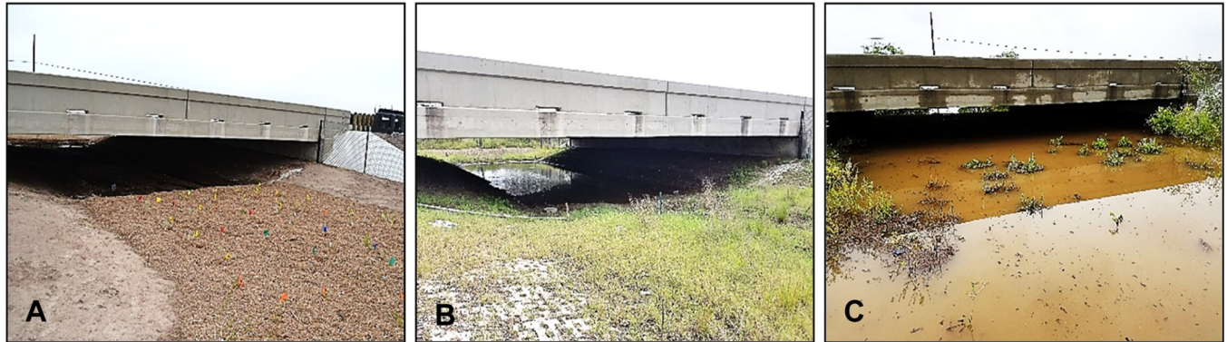
Fig 5. Water inundation at one wildlife crossing structure (bridge: Below grade), located on State Highway 100 in Cameron County, Texas, occurring between January 2018 and May 2019. Water levels depicted: little to no water (A); intermediate pooling of water (B); full of water (C). Reprinted from [40] under a CC BY license, with permission from A. D. Rivera Roy, original copyright 2020.
