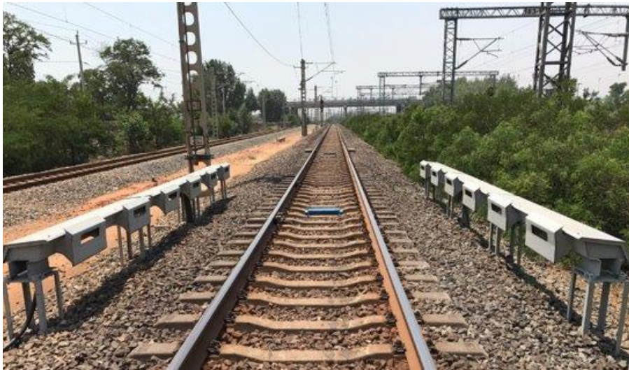
Figure 1. TADS system on the side of the railroad track [5]
